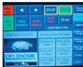
touchscreen control panel
